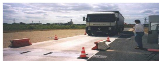
Weight in motion (WIM) overload vehicle detection system {Source: Low Speed WIM using load cell wheel scales in a concrete platform (Châlon s/Saône, France).}
